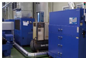
Capture fume generated during later sheet metal processing
