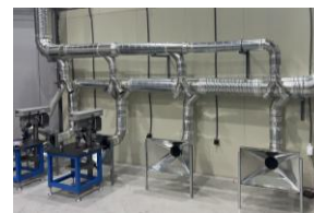
Dust collection from asbestos processing
