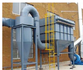
SAND BLAST pretreatment cyclone
