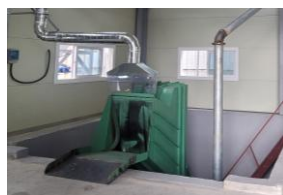
Dust collection from waste grinding
