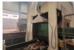
Dust collection from waste wood shredding
