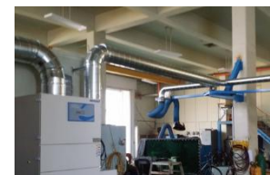
Welding fume capture
