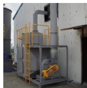
Chemical blending facility CACT
