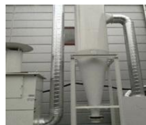
Abrasive, polishing facility
